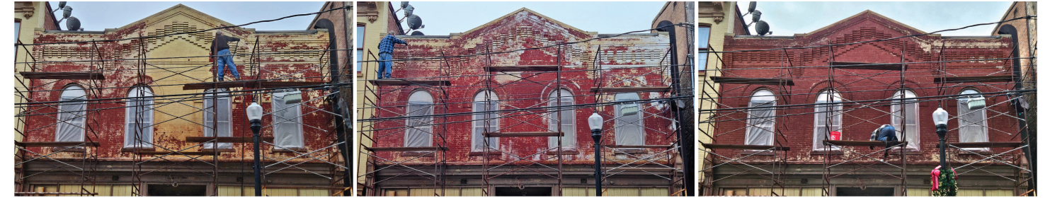
Thomas Shultz, historical masonry specialist, strips a century's worth of paint off of the brick Victorian façade at 240-242 W. King Street. Work continues to progress in restoring the historic architectural character of this building, funded in part with Façade Improvement Grant funds sponsored by the High Foundation.
